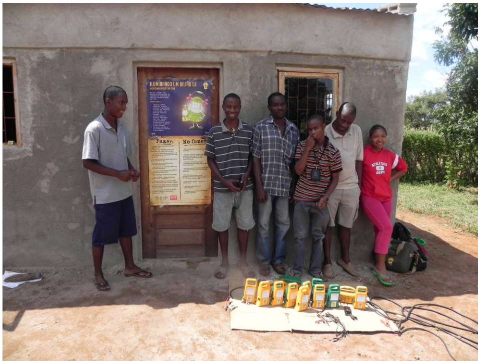
The lanterns are connected to the panel, and the instruction poster is on the door.
