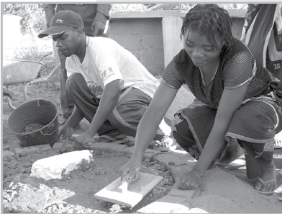
Producing a slab for a latrine of the kind in which a tree will later be planted
