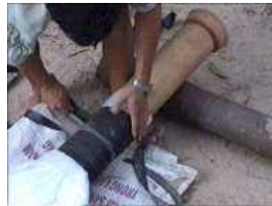
Photo 5. Wrapping the rubber bands around plastic tube where it overlaps the pipe
