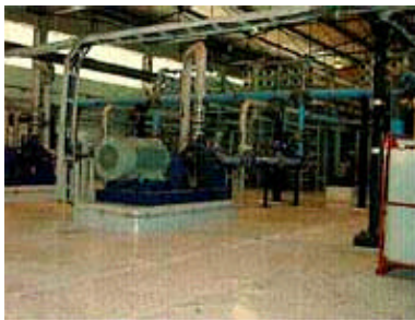
Fig 7: The desalination plant and high-pressure pump
